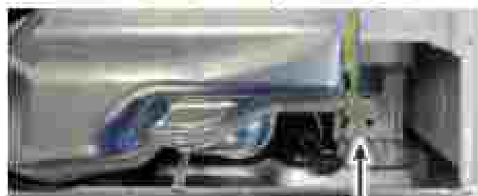
High-Limit Thermostat, Thermal Cutoff, & Heater Area
