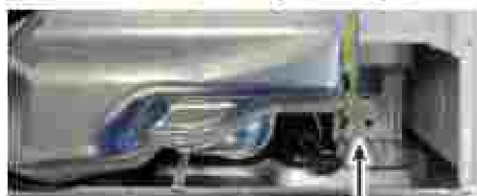
High-Limit Thermostat, Thermal Cutoff, & Heater Area
